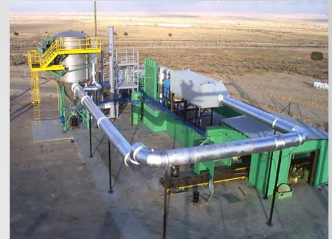
APE 1236 Rotary Kiln Incinerator at Tooele Army Depot
